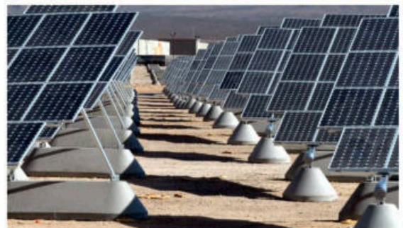
MONOCRYSTALLINE MODULES ON GROUND-MOUNT STRUCTURE, SCHEDULE ITEM 01
