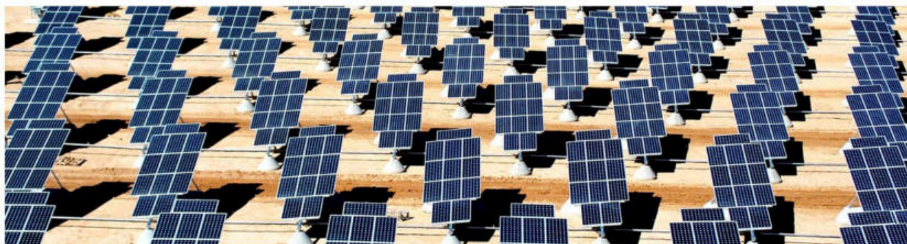
GROUND-MOUNT ARRAY OF THE KIND A PUMP CONVERSION IS BUILT ON
